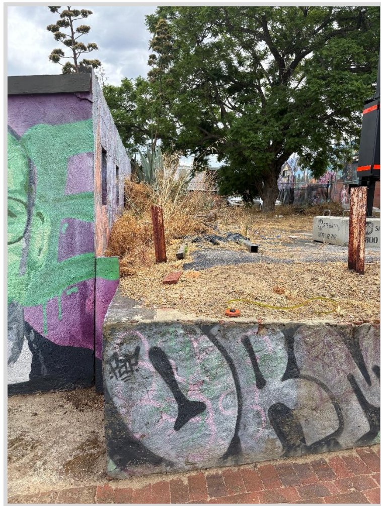
Figure 6: Displays the retaining wall from the side which is a height of 1 metre.
