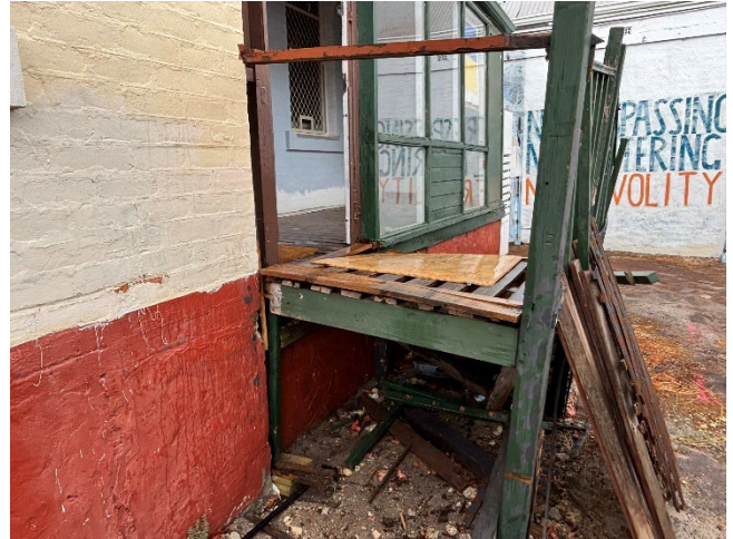
Figure 5 9 King William Street poor condition of entry ramp to verandah Source: Urbis 2026
